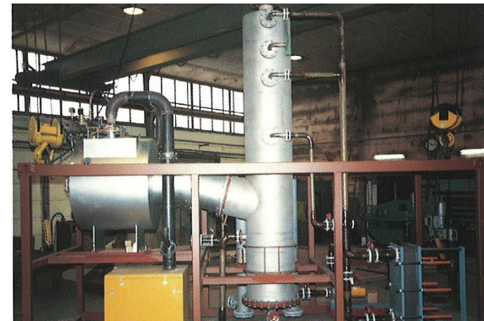
Skid-Mounted CF Burner with Quench Tower
